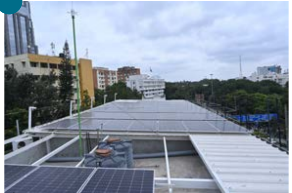
Harnessing solar power
